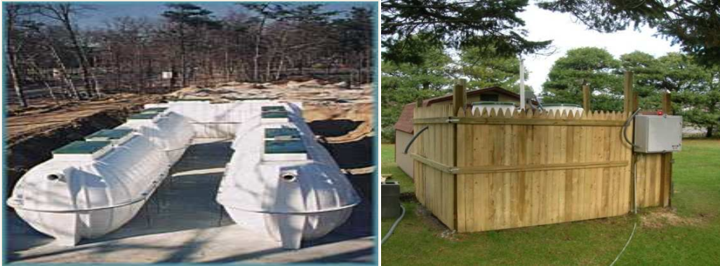
Figures 2a & 2b: The above left photo is of a preliminary below ground system and the photo to the right is of an operating above ground SBR system.
