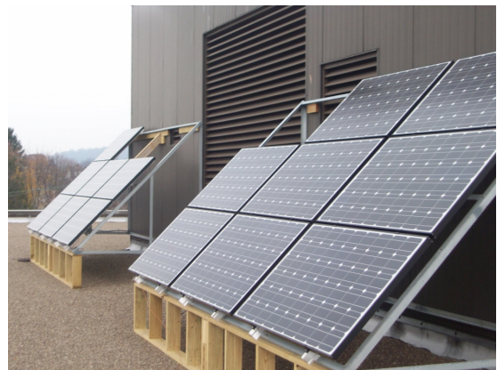
Side Photo: The 3.1 kW Photovoltaic (PV) System on the roof of the Heim building.
